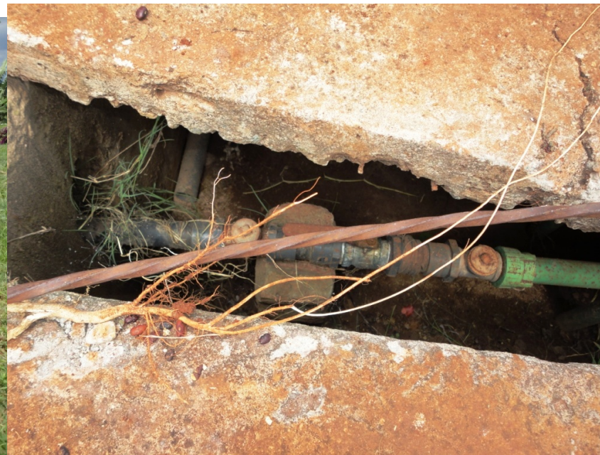
Biogas pipeline from digester to kitchen
