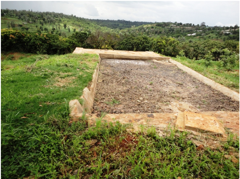
Wastewater post treatment stage
